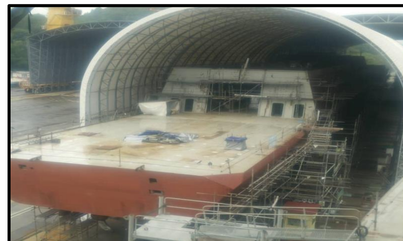
Aft deck with helicopter hangar
