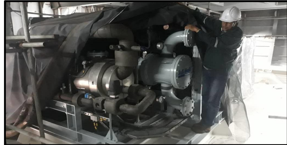
Chilled water plant installation
